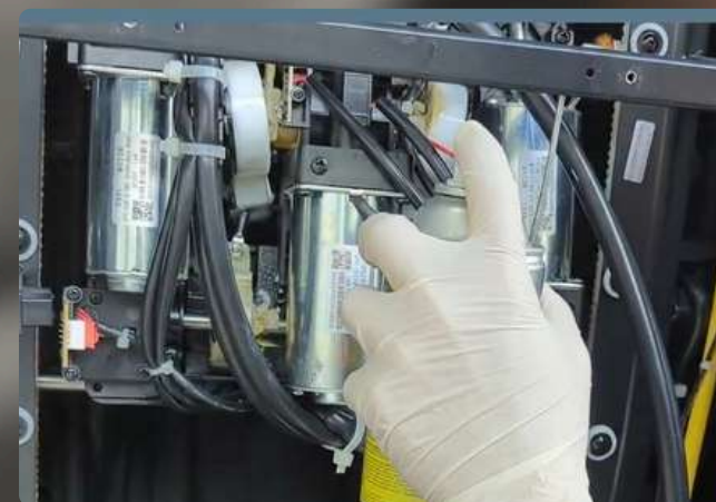
Motor Lubrication & Inspection [Every 12 th Month]
